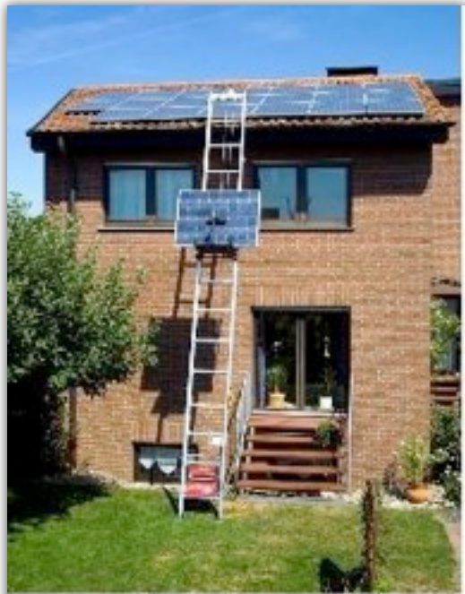
Solarlift Inclined to roof
