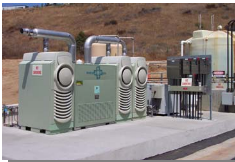
Three renewable-fueled Capstone C30 MicroTurbines installed at the SEJPA's Water Reclamation Facility.
