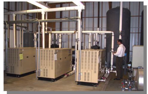
Ben Erpelding, Energy Engineer for the SDREO, inspects Dramm & Echter's cogeneration system.
