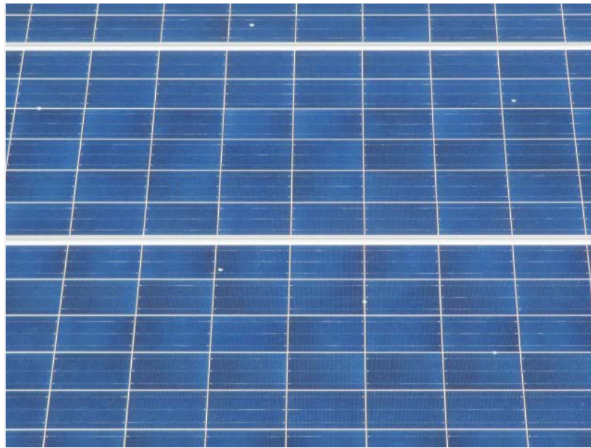
Photovoltaic solar power field at Volkswagen plant in Chattanooga, Tennessee
